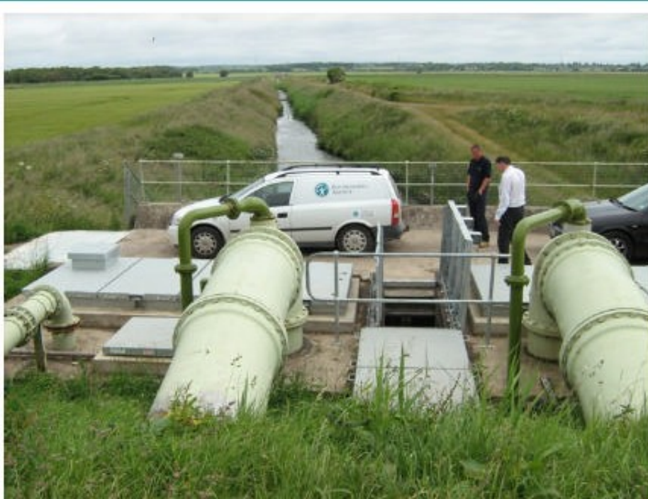
(Hey Cop Pumping Station – pipes and inlet channel)
