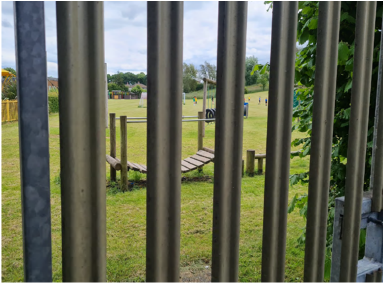
Palisade Fencing and Gates to be replaced and re-aligned
